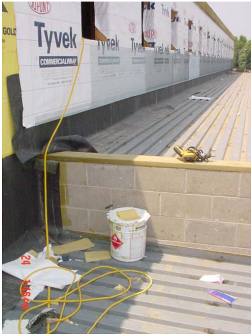
A 5-gallon pail is not a stairway
