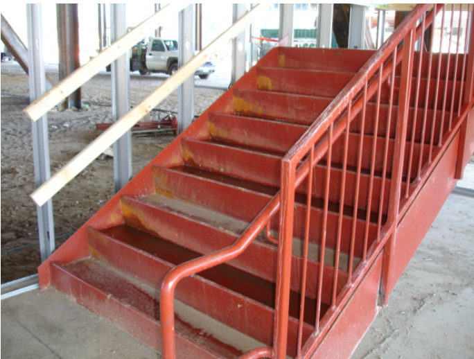
Stairway pans need to be filled
