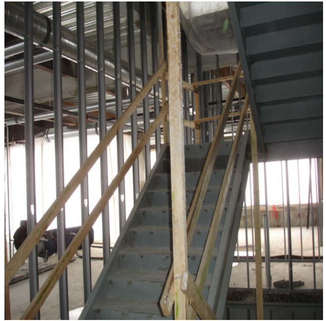
Handrails need to be in place
